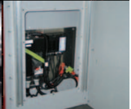
Electrical node with access panel
