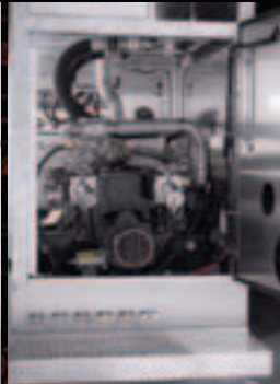
Full access to pump house
